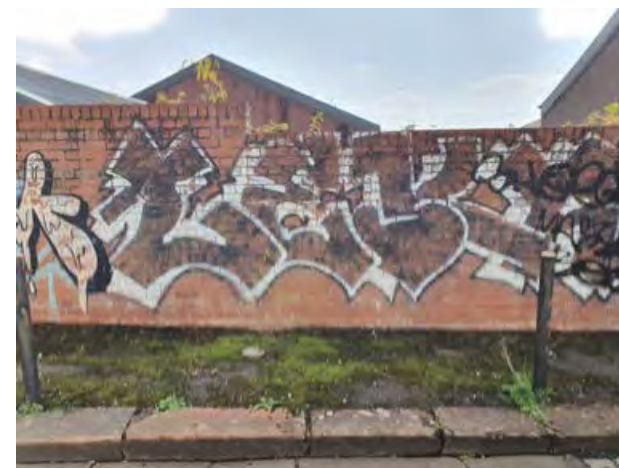
9.20 Illegal graffiti on Backhouses Walk
