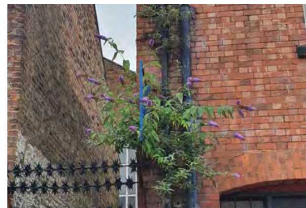
9.11a Example of poor maintenance on Crosby Street
