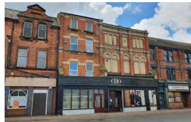
9.17 Examples of poor shopfront design, vacancy and changes to fenestration causing harm on Lonsdale Street
