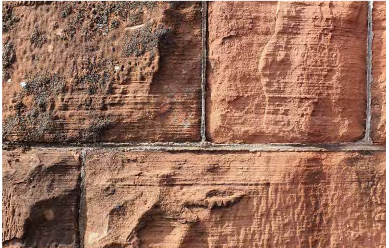
9.12 Inappropriate hard mortar leading to stone decay
